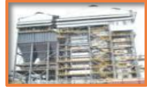
CPP-50 MW Installation
