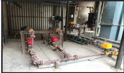
LAFR System in Line-3
